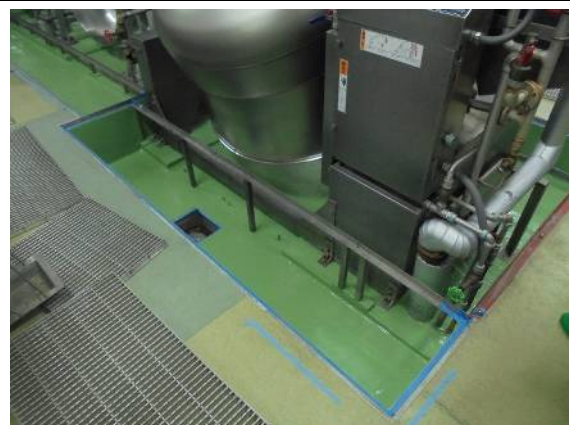
IM-38 蒸気配管
